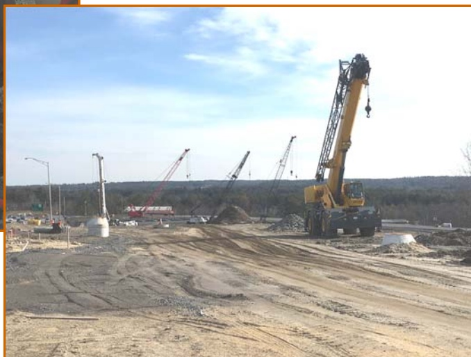
BELOW: FUTURE NH ROUTE 102. CRANES AND DRILL RIG, LOOKING EAST TOWARDS THE BRIDGE
