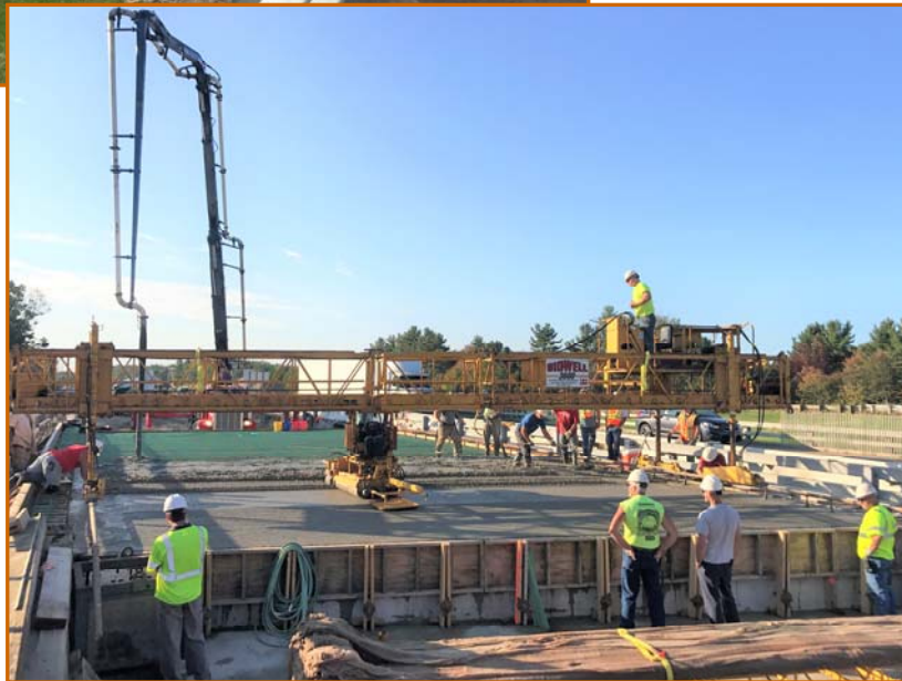
RIGHT: BRIDGE DECK POUR ON THE I-93 NB BRIDGE OVER STONEHENGE ROAD, FACING SOUTH..
