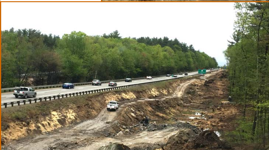
LEFT: AREA CLEARED FOR FUTURE WIDENING, DETENTION BASINS, AND AS A TEMPORARY ROAD FOR CONSTRUCTION ACCESS FOR CONTRACTORS.
