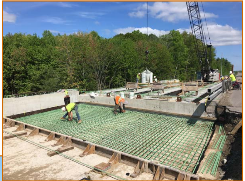
RIGHT: WORKERS TYING REBAR INTERSECTIONS ON SB BRIDGE OVER STONEHENGE ROAD APPROACH SLAB, FACING NORTH
