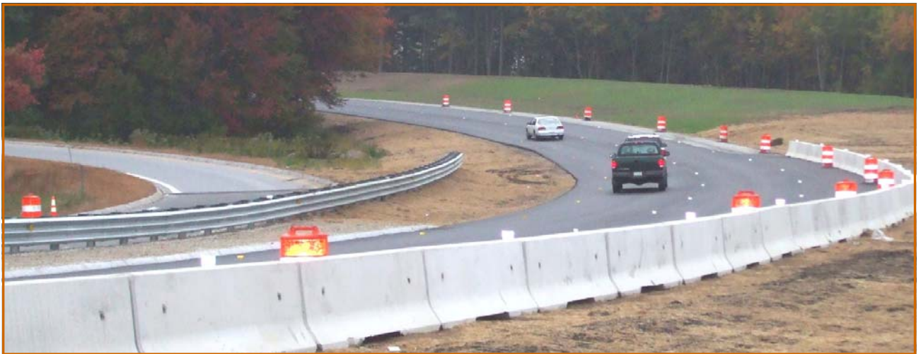
Existing Southbound off and on-ramps adjacent to partially constructed SB on-ramp (future alignment)
