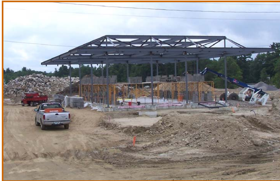
EXIT 2 BUS TERMINAL STRUCTURE APPROXIMATELY 6,000 CUBIC YARDS OF ROCK (MORE THAN 10,000 TONS) HAVE BEEN EXCAVATED FROM THIS SITE. THIS ROCK WILL BE CRUSHED AND REUSED IN THE PROJECT. AS OF AUGUST 1, 2007, THE PROJECT WAS 24% COMPLETE.
